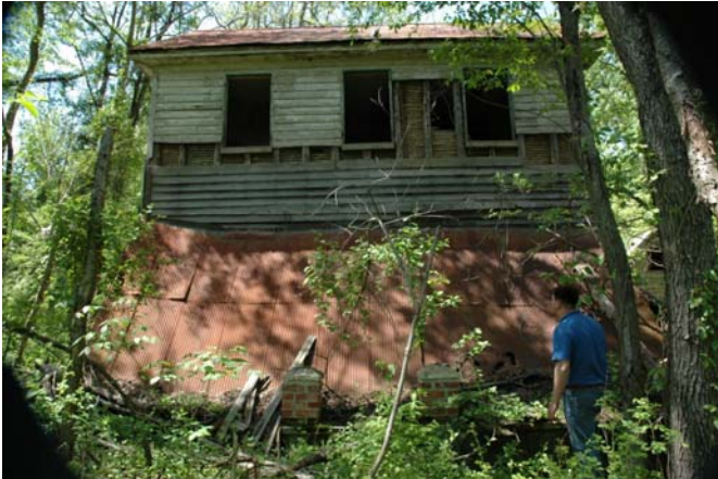
Front façade of house at Wilson Warfield Site 2, with collapsed front porch.
