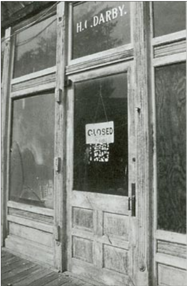
The Darby Store, built in 1910, is a typical two-story front gabled store in Montgomery County. The transom windows, display windows, and entry are important storefront elements that should be preserved. (Beallsville, MD)
