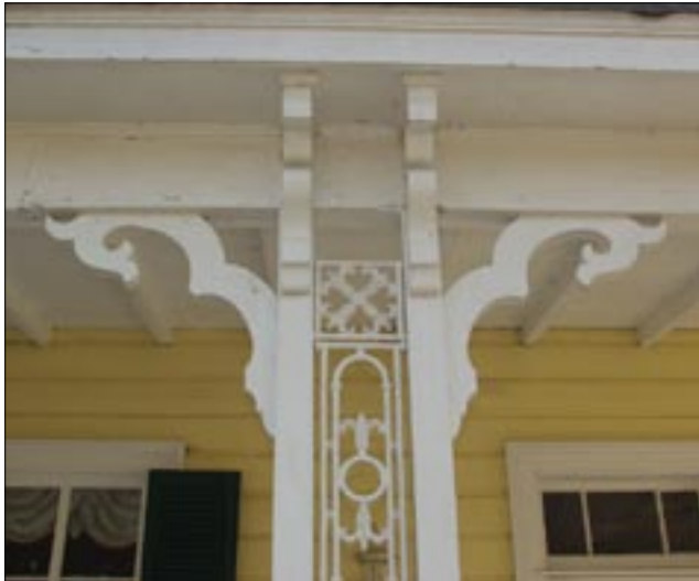
Guideline 1.1: A column bracket and associated moldings are character-defining features and should not be altered or removed.
