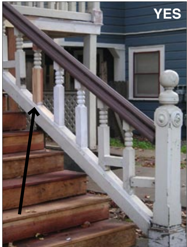
Guideline 1.4: It is appropriate to repair deteriorated building materials by patching, piecing-in, consolidating or otherwise reinforcing them. It is important to assess the cause of the damage and take steps to address the conditions that led to the deterioration.
