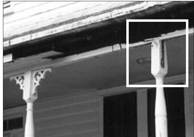
Guideline 1.8: It is appropriate to reconstruct a missing architectural element. In this case the missing bracket can be reconstructed based on the existing bracket.
