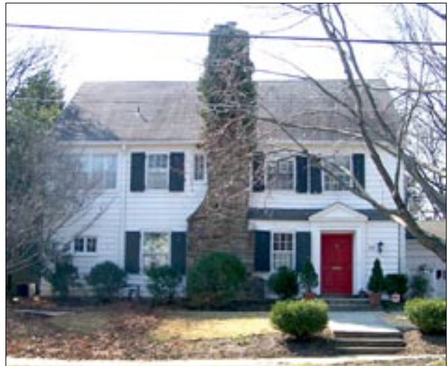
Guideline 6.1: Chimneys are important elements of a building and should be preserved. (Chevy Chase Village, MD)
