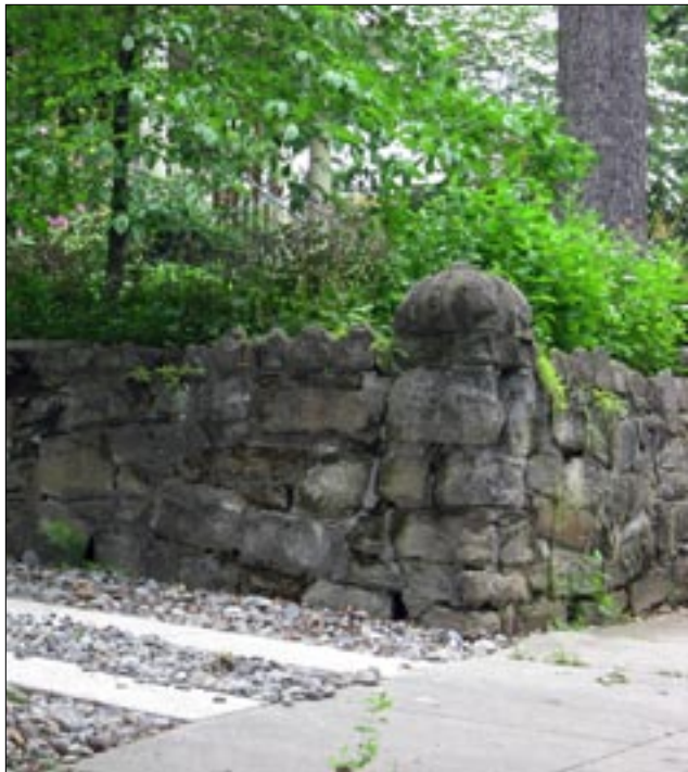
Guideline 13.1: Replace only those portions of a retaining wall that are deteriorated.
