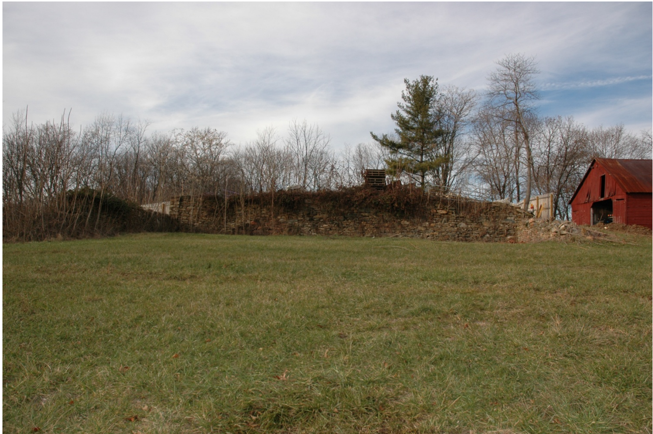
#15-17 Brandenburg Farm, Rubblestone Foundation of Former Bank Barn. Note Corncrib/Granary to the right. Sandra Youla, 12.18.2007
