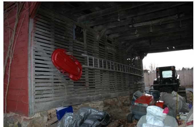
#15-17 Brandenburg Farm Corn Crib and Granary, Northeast Façade and Interior Wall of Corn Crib, with loosely-spaced narrow wood slats, Sandra Youla, 12.18.2007
