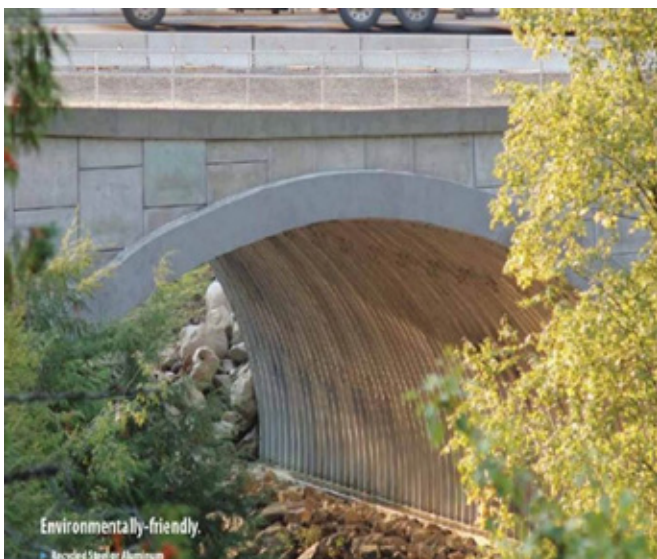
An example of a bottomless culvert, which is recommended for parcels 131 and 133
