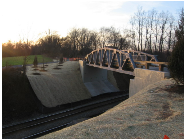
DTE designs and constructs transportation improvements, such as the Mouth of Monocacy Road Bridge, 2009 Maryland Quality Initiative Award of Excellence recipient .
